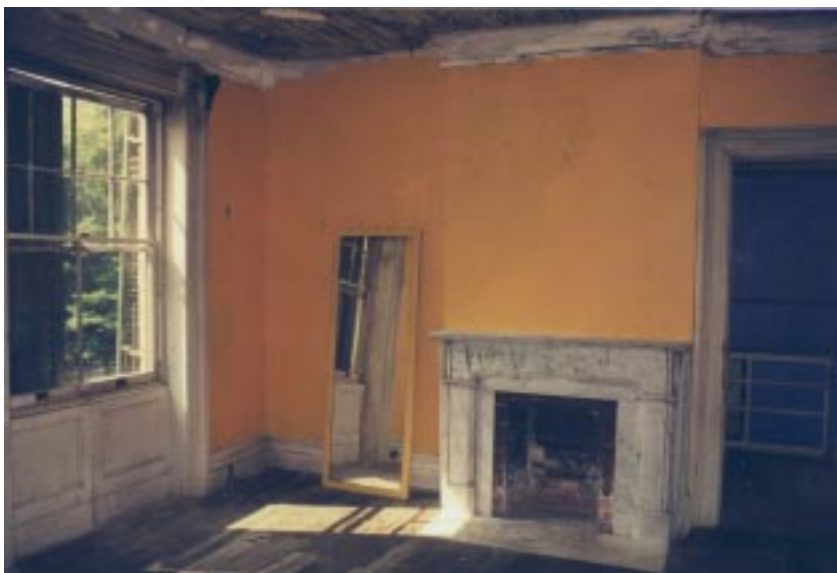
Above right: The northwest corner of Mrs. Kinkead's Bedroom. The marble chimneypiece, although of the same style as that in her Morning Room, is smaller. To the right in the photograph is a closet. Note the double panel apron under the window to the left and the damage to the run plaster cornice.
