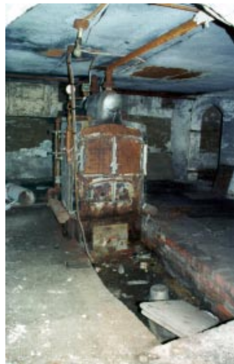
Maple Grove was retrofitted with a central coal-burning furnace to supply steam for radiators in the house.
