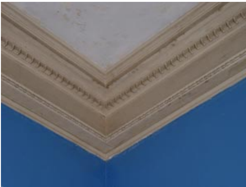
Crown molding in Passage is carried through into the Stair Hall and Library. Note the graceful relief of the patterning. The wood cornice remains largely intact.
