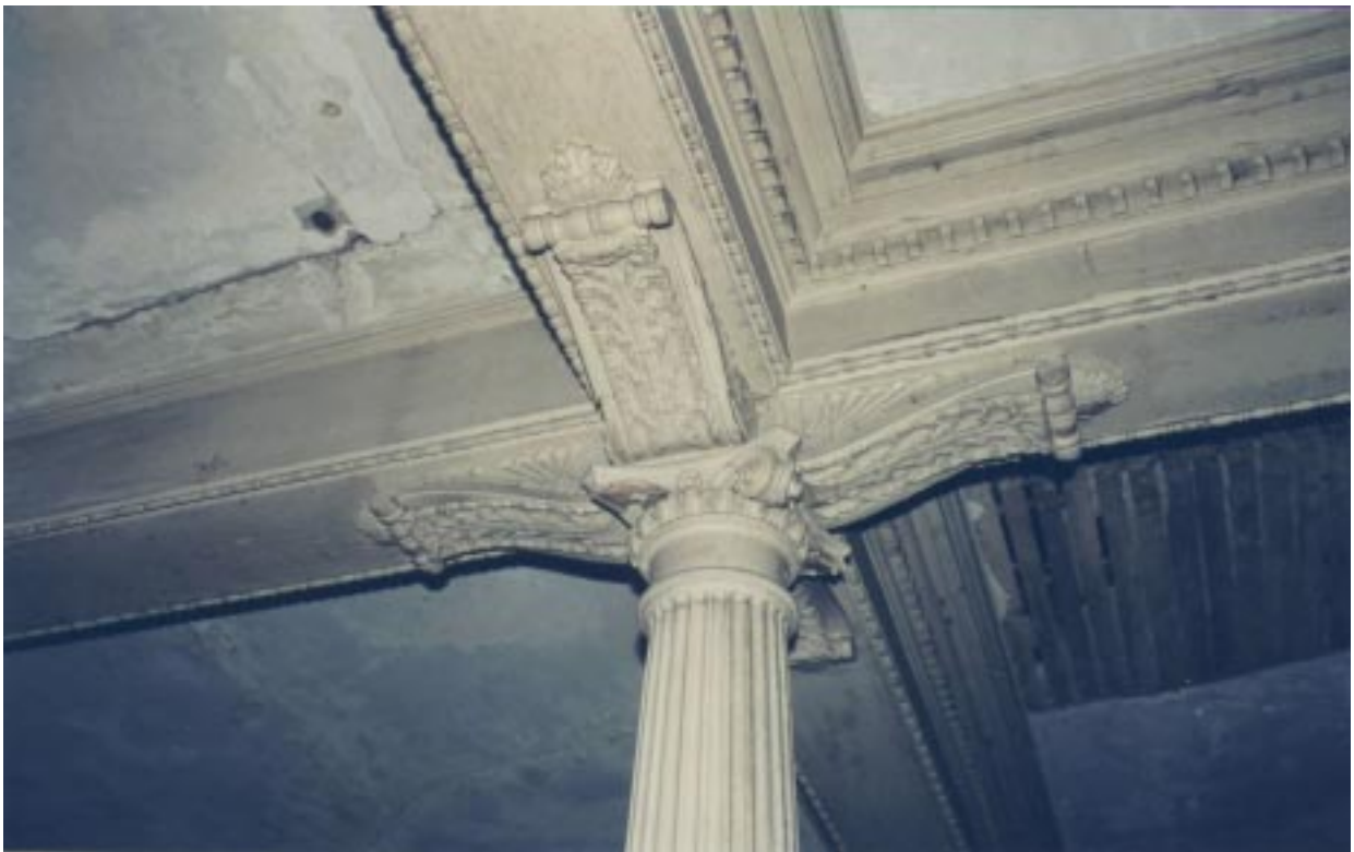
The fluted columns are crowned by a version of Composite order capitals with small Ionic scrolls below larger horizontal brackets in the shape of acanthus leaves. They appear to support the beams, which reflect the profile of the cornice. The woodwork is quite delicate and must be restored in several areas.
