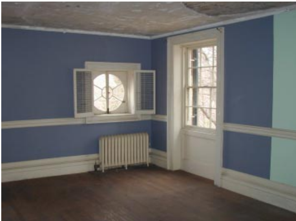
Northwest corner of North Wing bedroom. Note the square-framed circular window and the apron beneath the north window. In the upper right corner, the plaster of the ceiling is missing.
