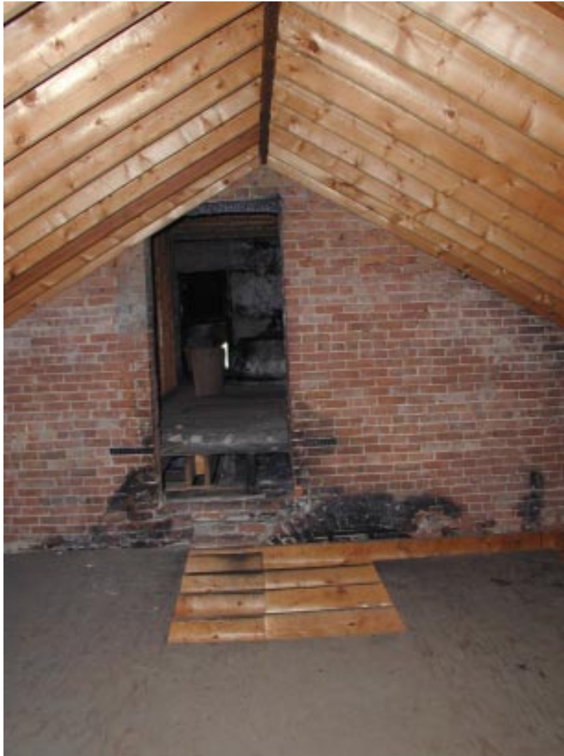
View from south attic room into main space up several steps. The service stairs ran up the brick masonry wall and arrived at the base of the opening. The floor opening visible in the photograph is used only to gain access to the attic spaces, not for the stairs.
