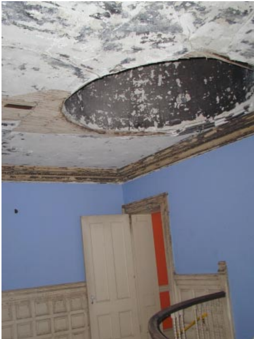
The northwest corner of the Upper Stair Hall is illustrative of the treatments existing today: the Colonial Revival paneled wainscotting, the curved balustrade, the Greek Revival architraves, the paneled jambs at the intersection of the main block and north wing, and the skylight opening.
