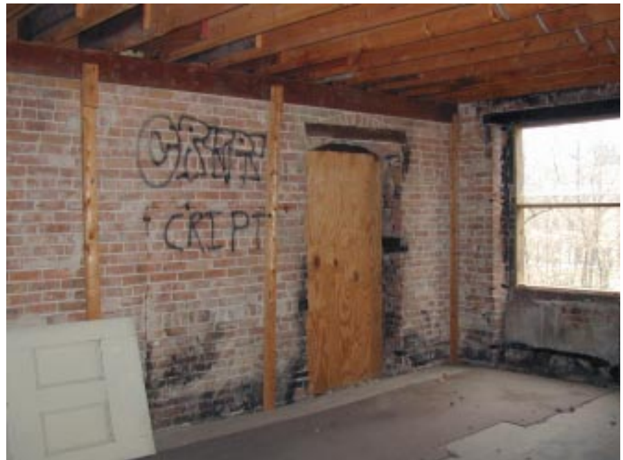
The east wall of the South Wing. Note the new wood ceiling joists. The door opening should be reconfigured as a window according to the 1891 plan.
