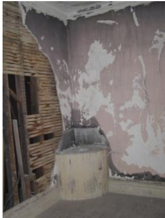
The small corner sink in the Guest Room has a marble countertop and backsplash with a curved wood-slat cabinet beneath. Note the condition of the plaster to the left. It should be replaced using the blueboard system as the damage is extensive.
