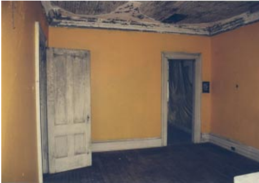
Right: The southwest corner of Mrs. Kinkead's Bedroom. The door on the right leads into the Morning Room and on the left leads out to the Upper Stair Hall. A considerable portion of the ceiling was damaged during the 1985 firefighting efforts.
