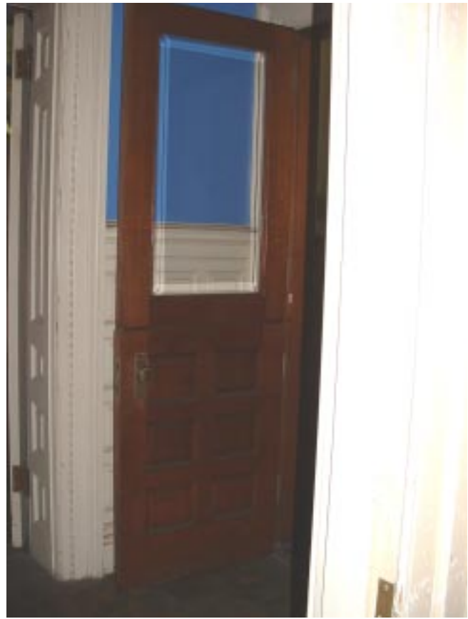
The inner vestibule doors are similar to the exterior doors except that they are split in the middle and latched, similar to Dutch-style doors. Note the door architrave with its attenuated bead.
