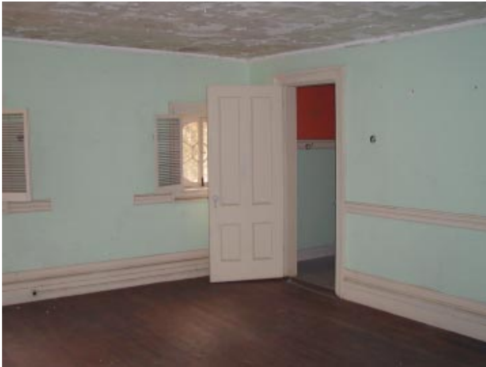
Southeast corner of North Wing with the bathroom. Note the tall very tall baseboard moldings, the break in the chair rail between the windows on the east wall and the four panel door.
