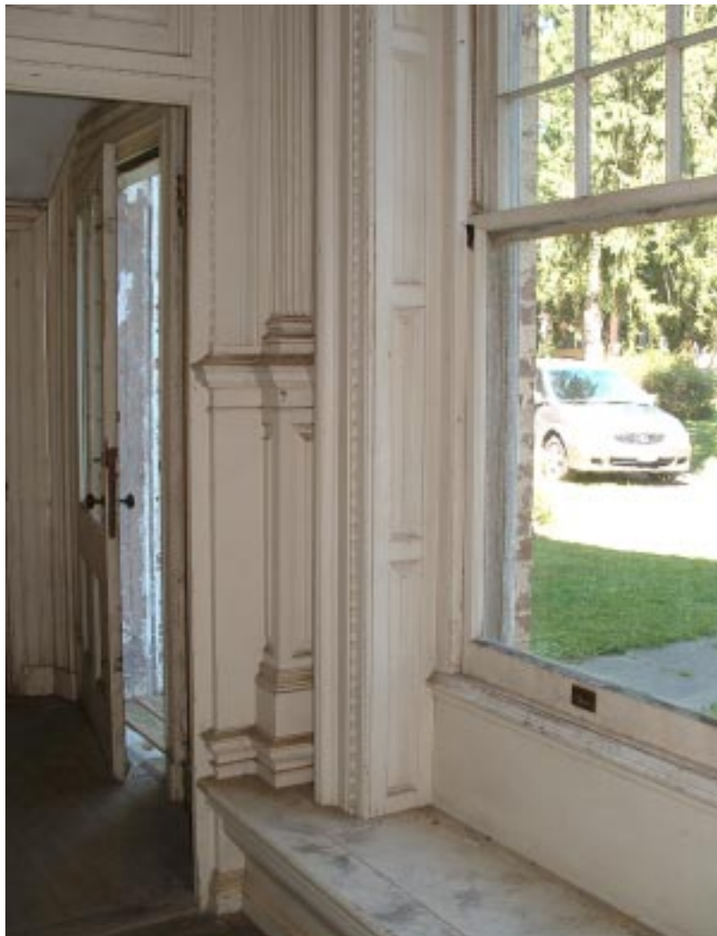
View into the back Vestibule past the east windowseat. Note the jamb panels. Although the east brick masonry wall is equal in thickness to those surrounding the other windowseat openings, the jamb panels are considerably narrower perhaps owing to the use of the fluted column seen to the left of the jamb. The partition between the Library and back Vestibule is only 2-1/2" thick.
