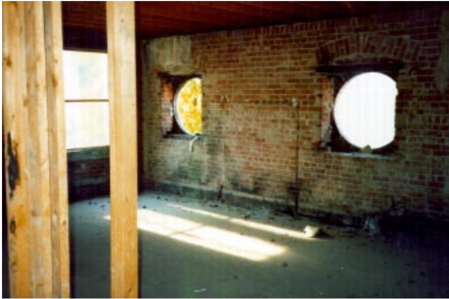
West wall of South Wing. Note the circular and square masonry openings made possible by the cavity wall construction employed at Maple Grove. All the windows should be restored and the blueboard system used to finish the room. A fireplace is located to the left of the double-hung window seen through the studs in the foreground.
